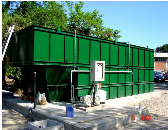
Moving bed bio reactor
